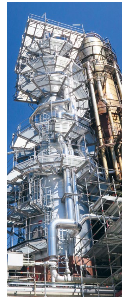
Neue Pre-Flash-Kolonne in Cressier.
